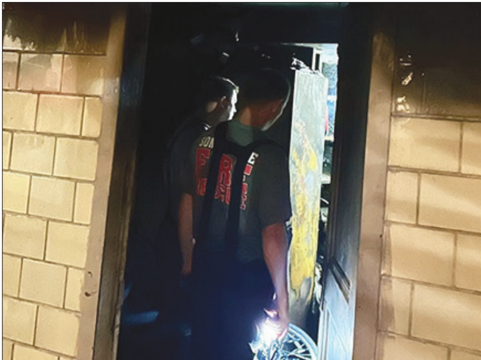
Firefighters inspect fire damage inside a second-floor apartment following Sunday's two-alarm fire. — Photos courtesy of the Somerville Fire Department
