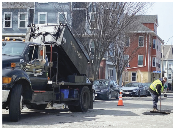
Pothole repairs being done on Highland Ave. last Wednesday afternoon. — Photo by Bobbie Toner
